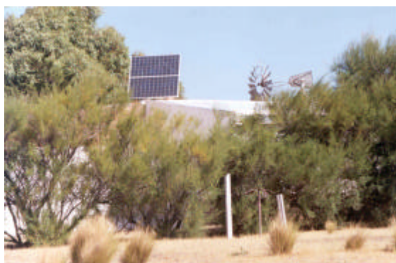
New solar panels installed, provide 100% sustainable energy at La Esperanza,
